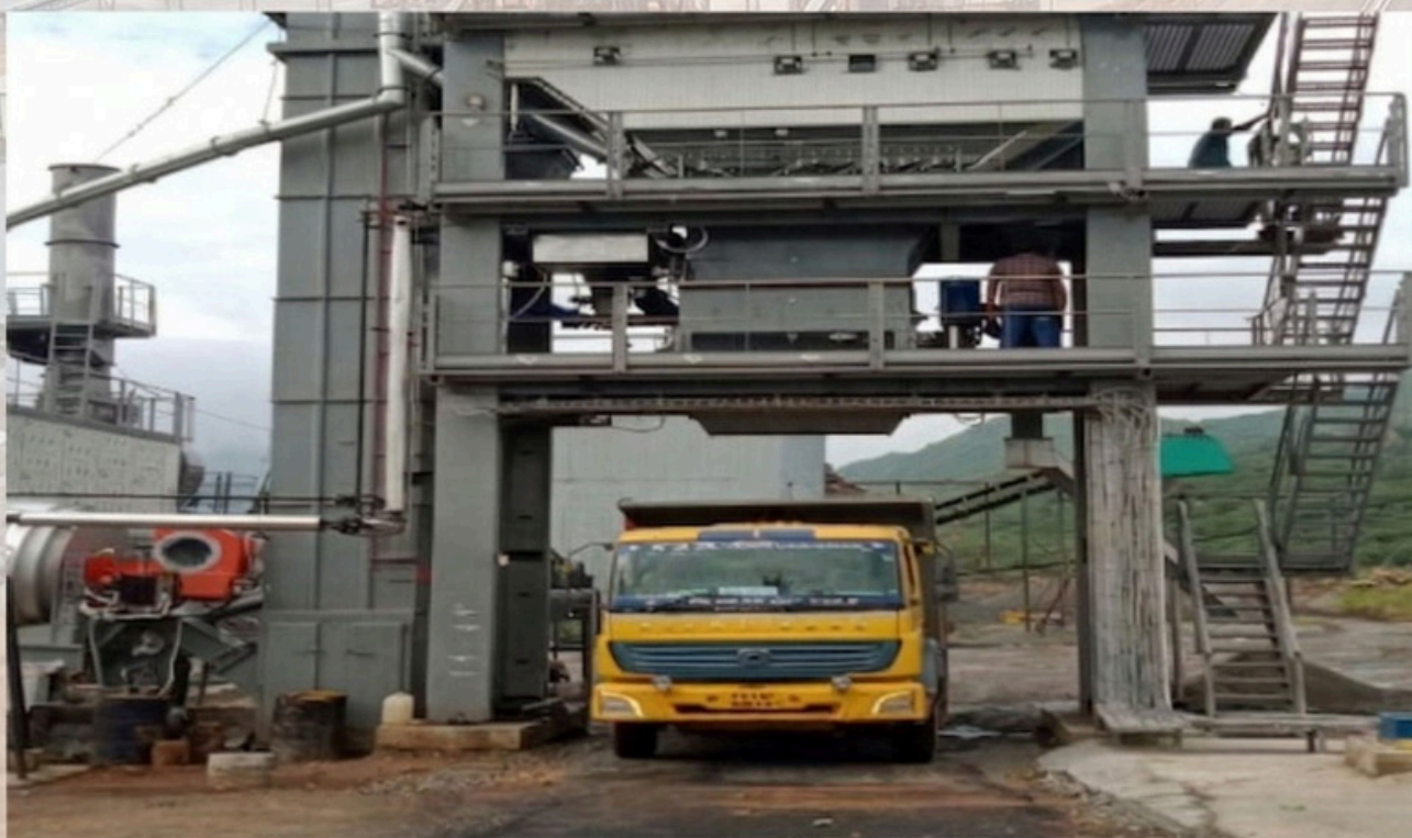
Hot Mix Plant Located Andipatti, Theni & Nagercoil
