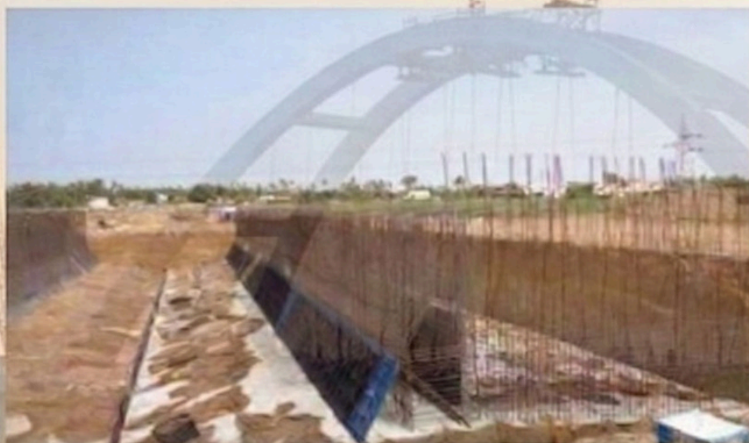
Major Bridge work across Narikulam Tank from Km.230/600 to Km.231/250 in Madurai - Kanyakumari section of NH 7
