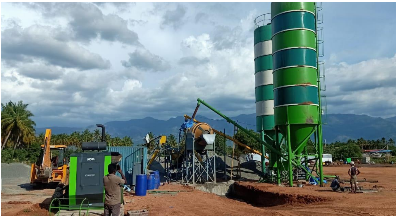
Ready Mix Concrete Plant
