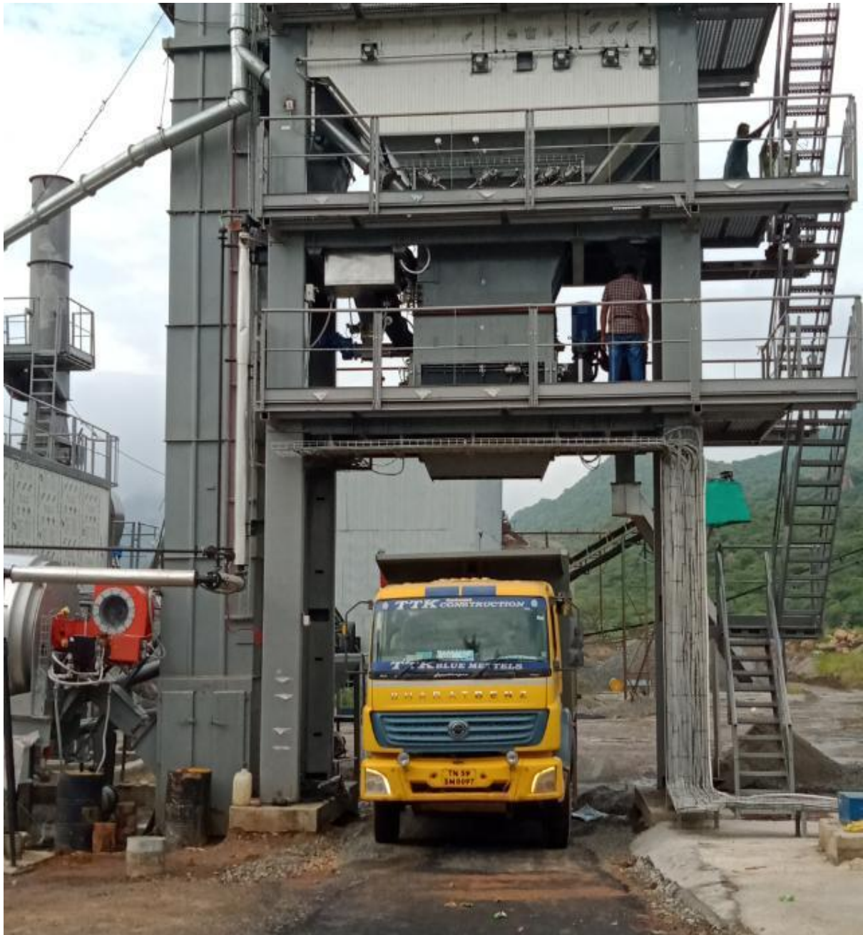
Hot Mix Plant
